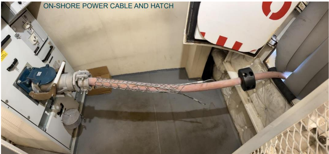
Figure 20 TWIN-Port III - On-shore power cable and hatch
